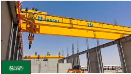
25T Double Girder Overhead Crane
