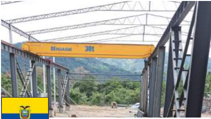
30T Double Girder Overhead Crane
