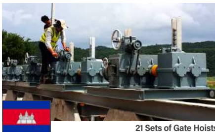
21 Sets of Gate Hoists
